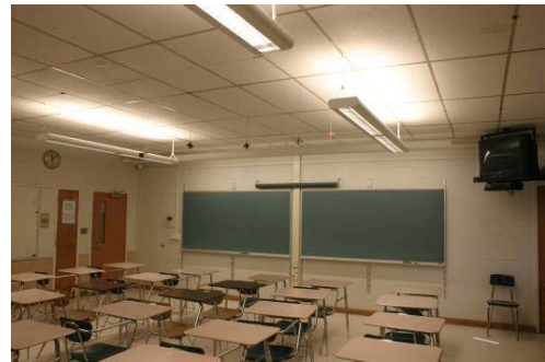
Figure 2: After retrofit with ICLS (General Mode and Whiteboard on)
